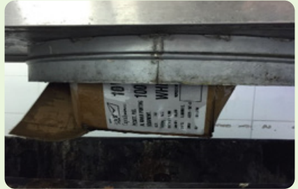
Inappropriate material blocking the garbage chute
