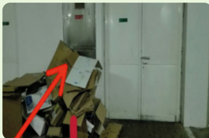
Waste material discarded inappropriately outside garbage chute
