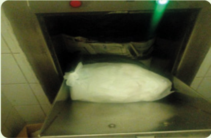
Blocked garbage chutes
