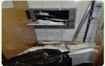
Blocked access and dirty waste rooms
